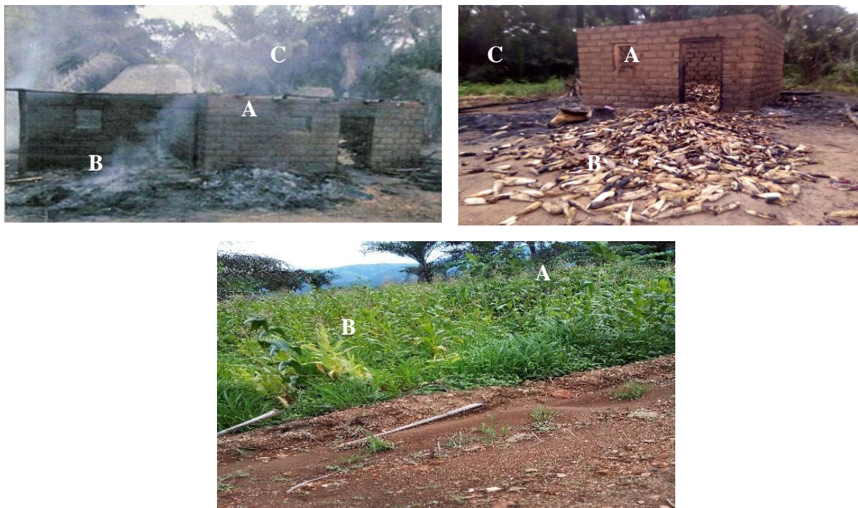
Photo 1: (A) burned house (B) burned properties (C) palm trees Date: June 12, 2021 at 2:02 p.m. Photo 2: (A) a house, (B) burned corn, and (C) a palm tree. Date: June 26, 2021 at 10:15 a.m. Photo 3: (A) healthy corn; (B) grasses that overshadow the corn, causing it to change colour. Date: June 12, 2021 at 2:02 p.m.
