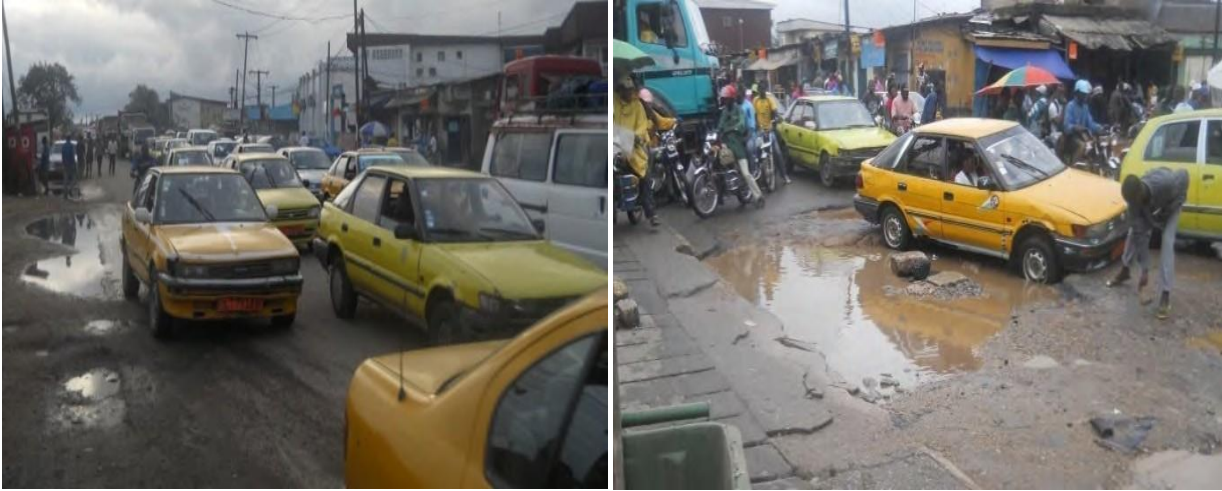
Photo 8: Large potholes at Akak 11 which has widen over time & a deplorable nature of the road especially during rainy season
