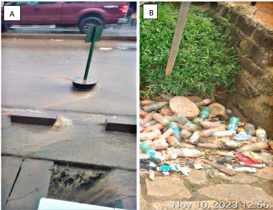
Plate 6: flash flooding (A) and blocked drainage systems (B)
