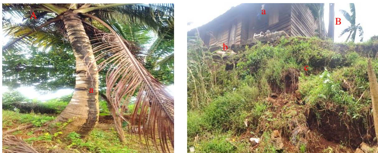
Plate 3: Evidences of soil creep (source: Eti November 2020)
