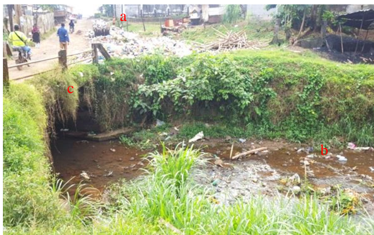
Photo 5: showing under sizing of a bridge at lower Mawoh.
