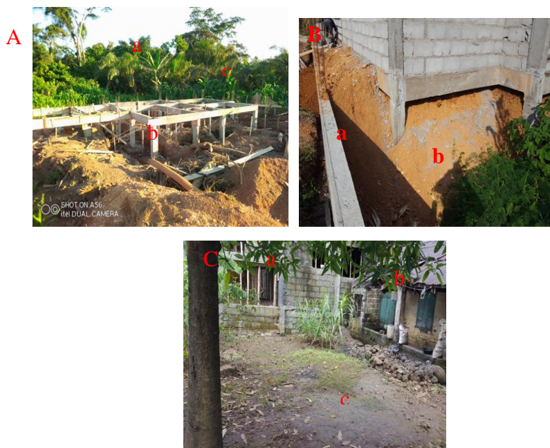
Plate 9: High foundation at Bonjo and clerks' quarters to cope with floods (Source: Eti November 2020)
