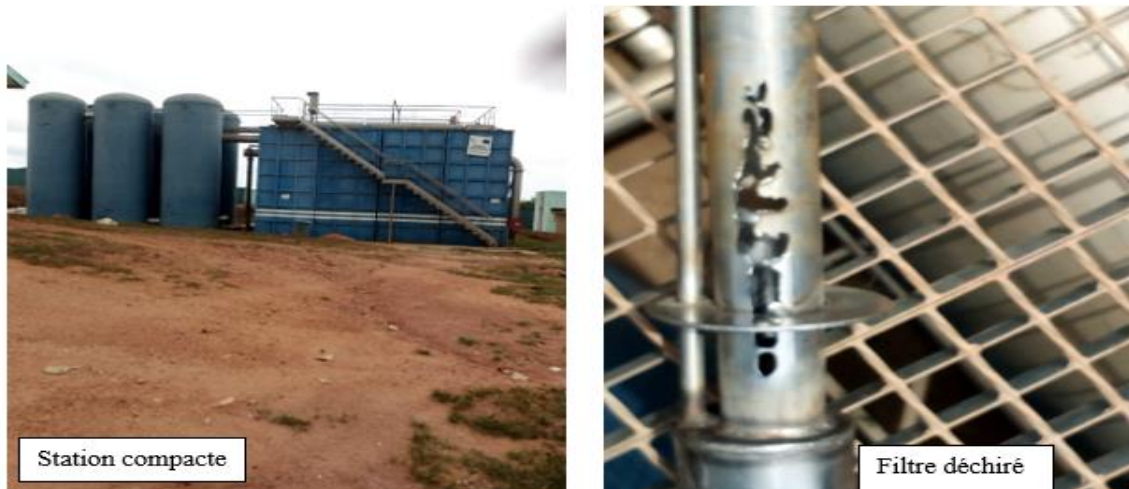
Figure 43 : Station compacte endommagé
