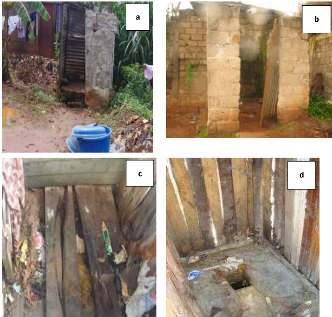
Fig. 36. Photos showing some unsafe latrines with discomfort found in the study area (a: dirty latrine built with metal sheet located in a flooding area; b: latrine with unfinished superstructure showing weak maintenance; c: unsafe latrine with a wood slab partially built and full pit continuously in used; d: dirty latrine with partially built superstructure) (Photos: Letah Nzouebet).
