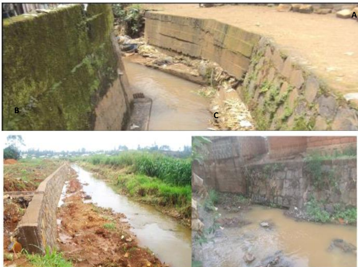
Figure 1: Channel straightening, embankment and channel reduction for land reclamation purposes ( Source: Fogwe, 2016).
